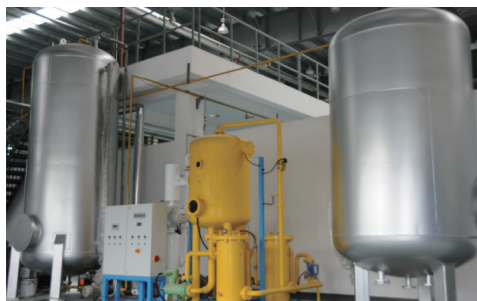
Advanced oil treatment system
