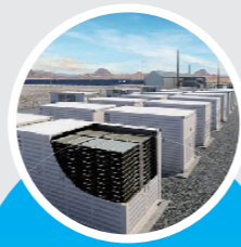
Containerized Energy Storage
