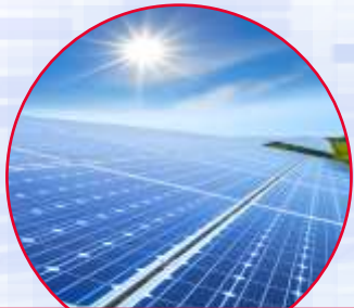
Photovoltaic power generation
