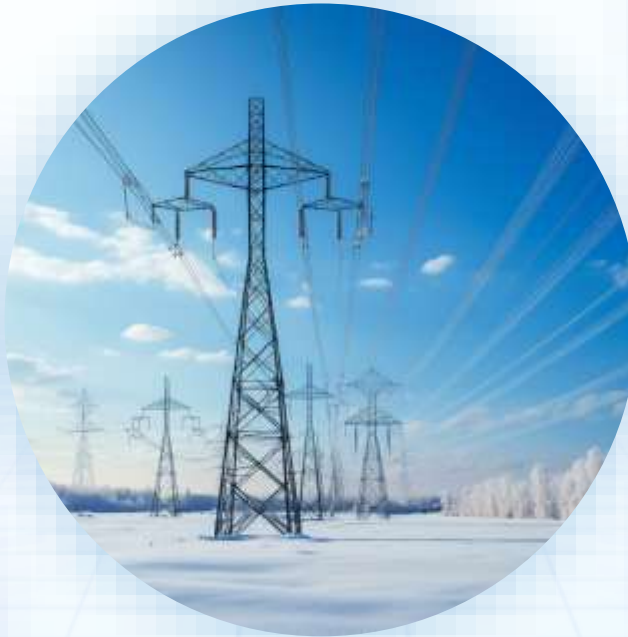
Flexible and conventional UHV DC transmission Flexible DC and flexible low-frequency power transmission
