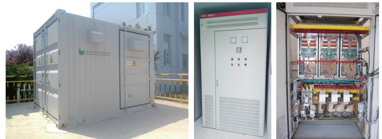
Baosheng Photovoltaic SVG
