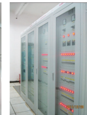
Control and Monitoring Panel
