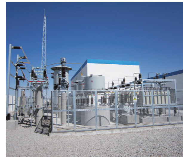
Photo of SVC Unit for Erlianhaote Wind Power Project of China Huadian in Inner Mongolia
