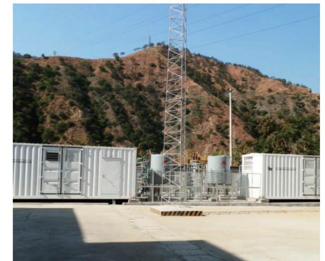
Photo of SVC Unit for the Electrified Railway of China Railway Chengdu Bureau
