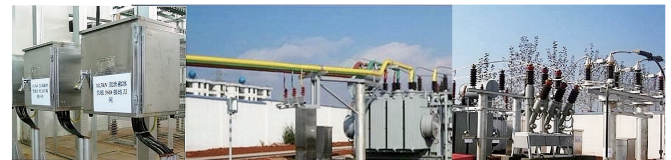
DC Ice-melting for Yunnan Power Grid
